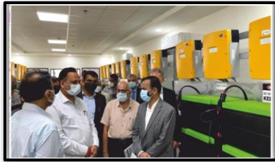
Shivalik Project Micro Grid Solar Power System Installed at Shivalik Grid in Delhi
