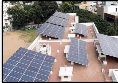
UPNEDA Offgrid Solar Project at UP govt. offices
