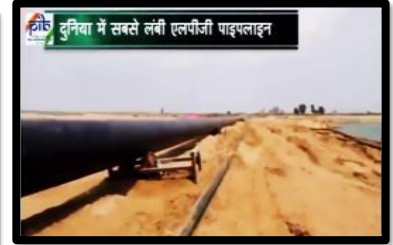
Kandla-Gorakhpur LPG Pipeline Solarizing a total of 158 sites on the country's longest LPG pipeline - spanning 2,757 Kms - from Kandla Port, Gujarat to Gorakhpur, Uttar Pradesh
