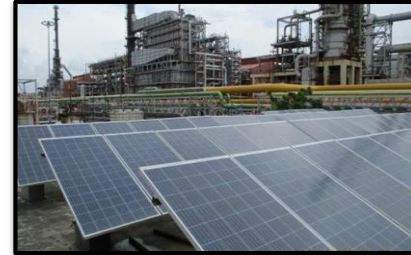
Rooftop Solar Project BPCL (Mahol Refinery)
