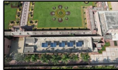
Akshardham Project India's First Portable Rooftop Solar Systems Installed at Akshardham Gandhi Nagar
