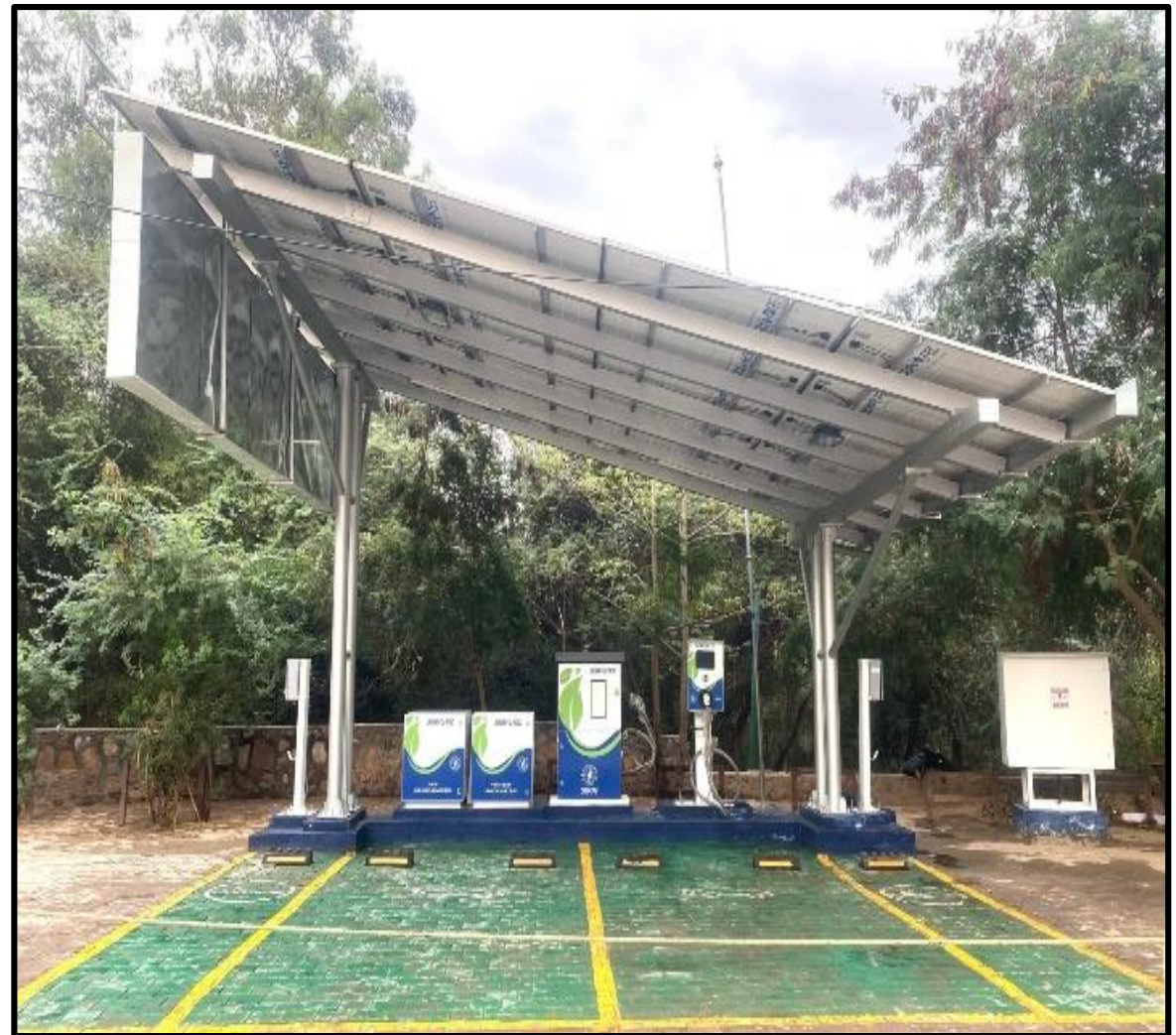
Solar powered EV Charging Carport
