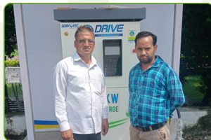
Gym Khanna Service Station BPCL Delhi
