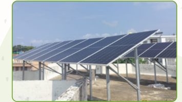
Glimpse of Sub District Hospital Tanakpur-100kw
