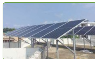
Glimpse of Sub District Hospital Tanakpur-100kw
