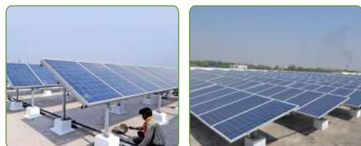
Carried out a mega project of 3MW at multiple locations across Chennai
