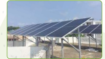
Glimpse of Sub District Hospital Tanakpur-100kW
