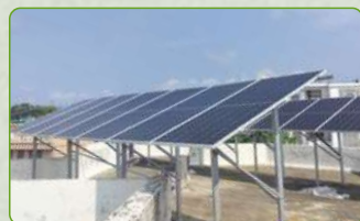
Glimpse of Sub District Hospital Tanakpur-100kW
